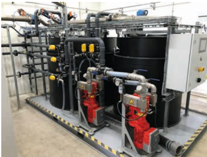
Depot in UK: 2 x TUnit MP Bio Machine room with 2 x VacUnit DP VX136-140Q, NeutraUnit, (AT and CNT tank)
